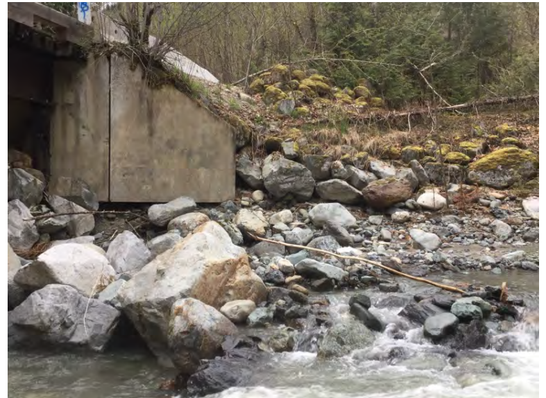
Upstream right bank riprap scour
