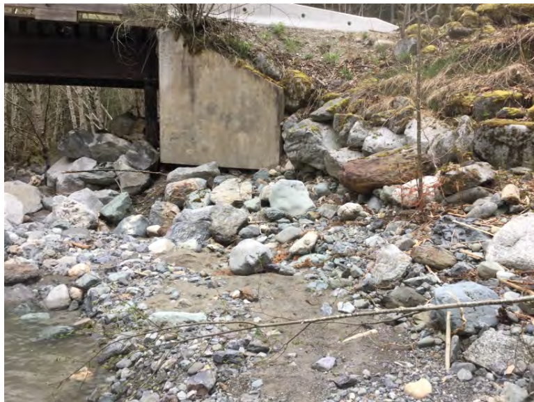
Upstream right bank scour
