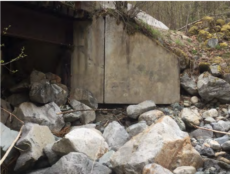
Upstream right bank ballast and wingwall scour
